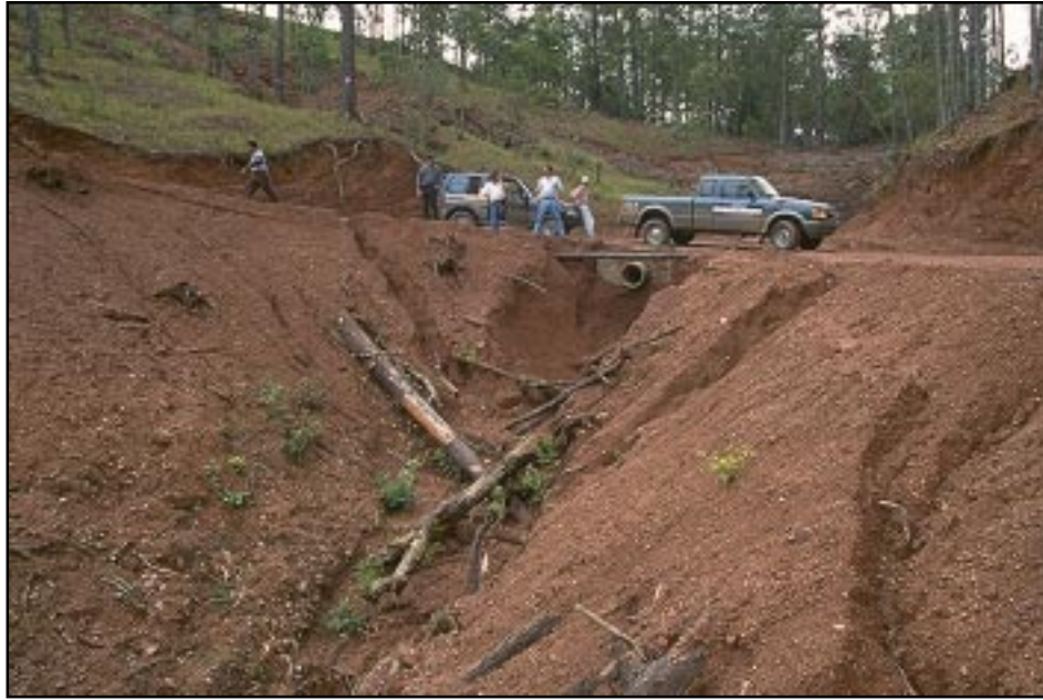
Photo 8.9 Avoid culvert outlets in the middle of a fill slope. Use culverts long enough to extend to the toe of the slope, or use headwall structures to retain the fill material and minimize the pipe length.
