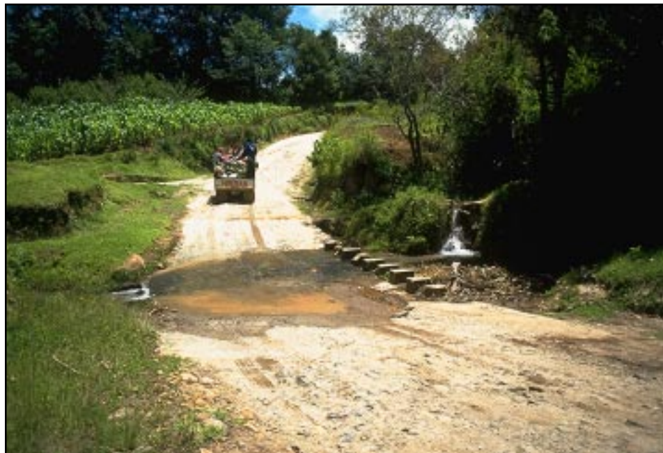
Photo 9.1 Use armored low-water crossings, fords, or drifts as often as possible to cross low flows in broad, shallow natural drainages, thus avoiding the use of pipes. Note that part of this reinforced driving surface needs repair.
