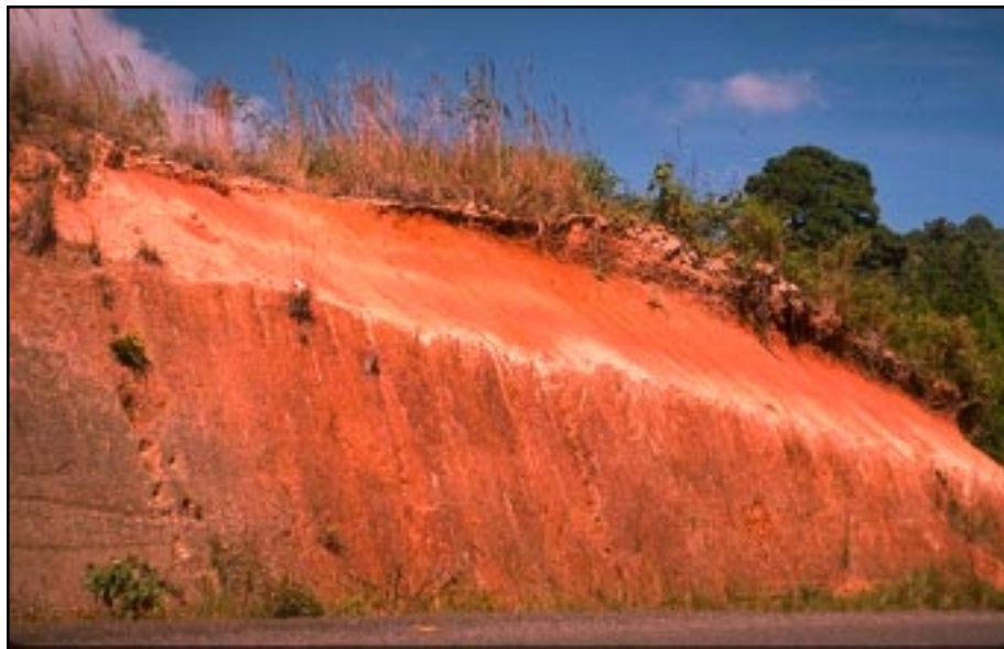
Photo 11.2 Construct cut slopes at a 3/4:1 or flatter slope in most soils for long-term stability. In well-cemented soils and rock, a 1/4:1 cut clope will usually be stable.
