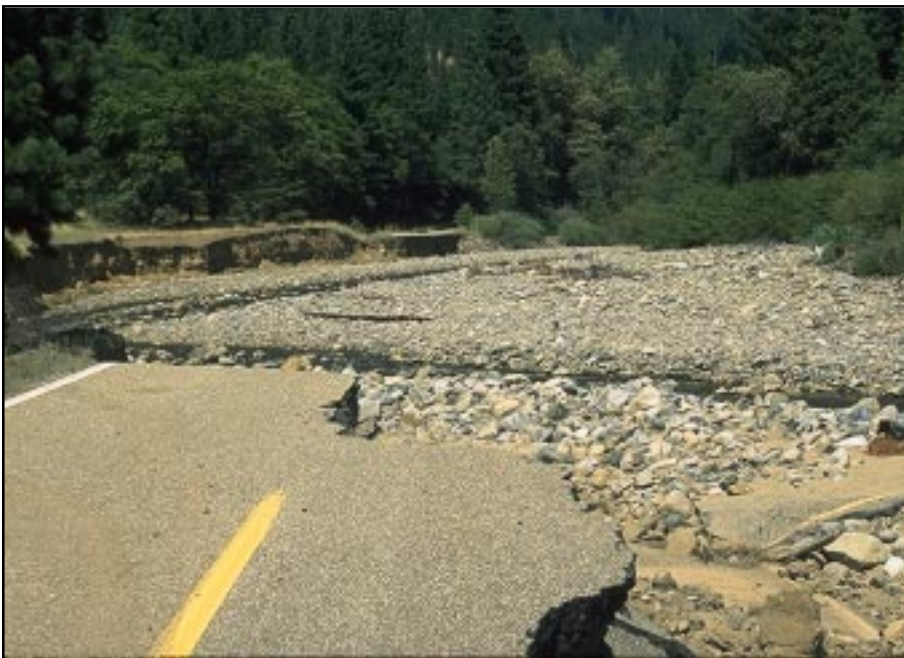
Photo 3.3 A poorly located road, in the hazardous flood plain area of a river, that has washed out during a major storm event.
