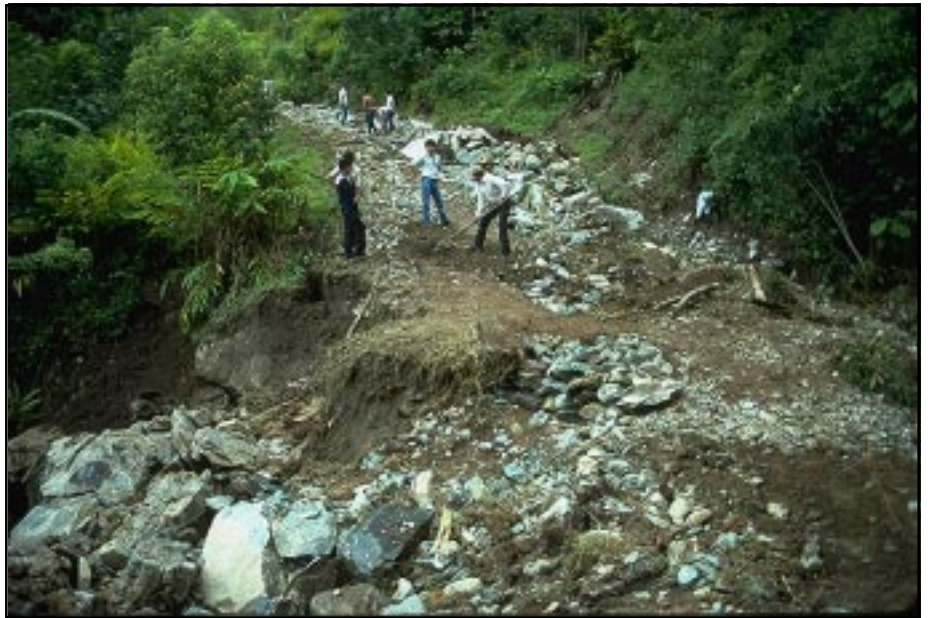
Photo 3.4 A road that has been heavily damaged during a storm because of an undersized, plugged culvert pipe and no overflow protection.
