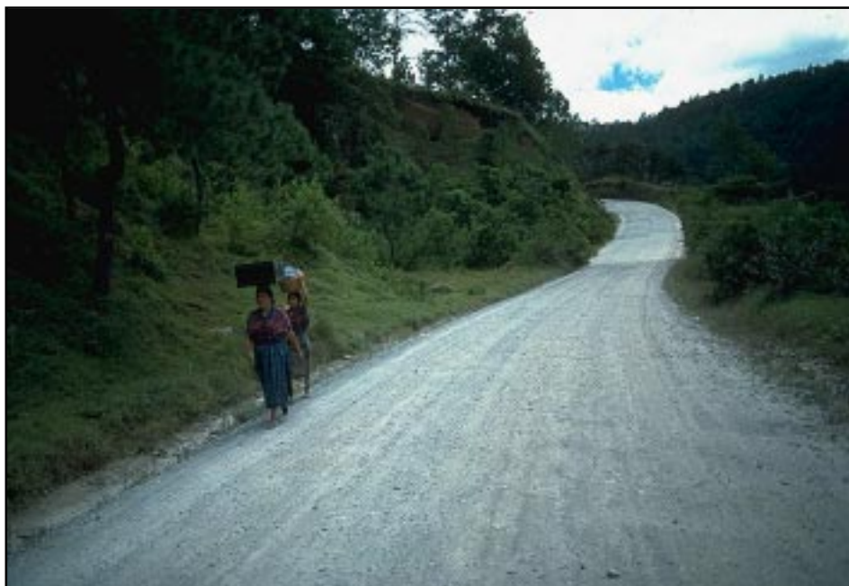
Photo 1.1 A minimum impact rural road that is well drained, has a stable driving surface, stable slopes, and is satisfactory for the user.
