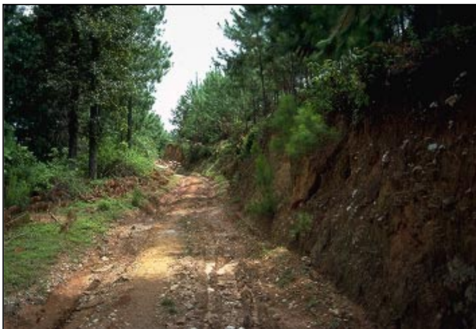
Photo 12.1 A rutting road caused either by soft subgrade soil or inadequate road drainage (or both).
