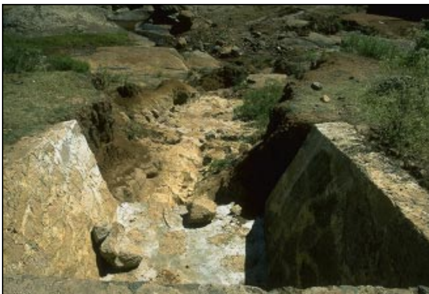
Photo 7.4 Add outlet protection and/or energy dissipators to prevent erosion and the formation of gullies.
